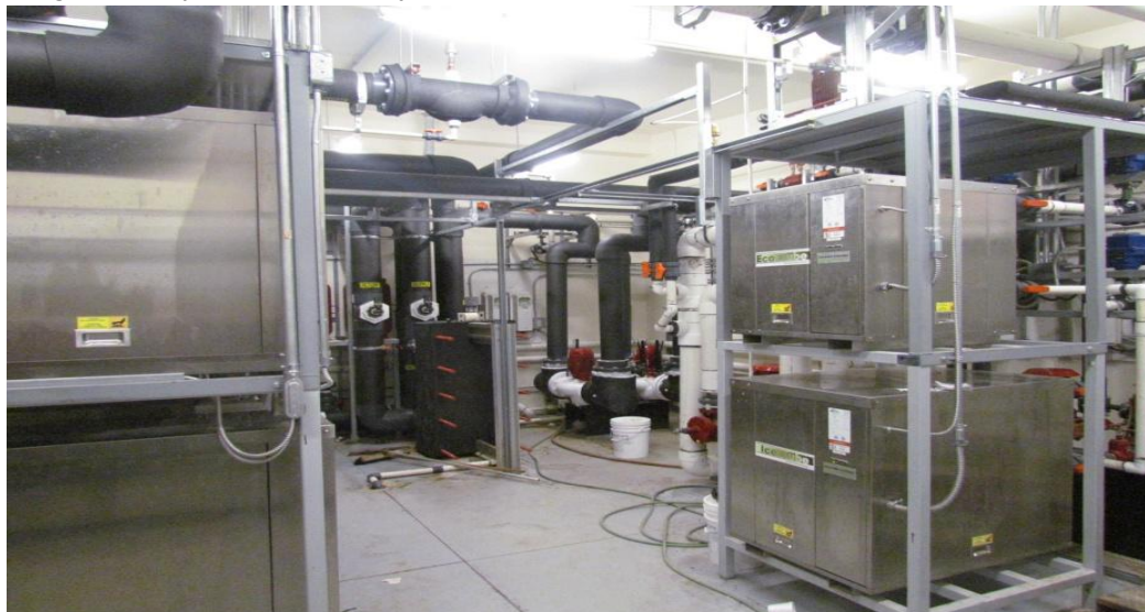
New geothermal systems at the Carberry arena
