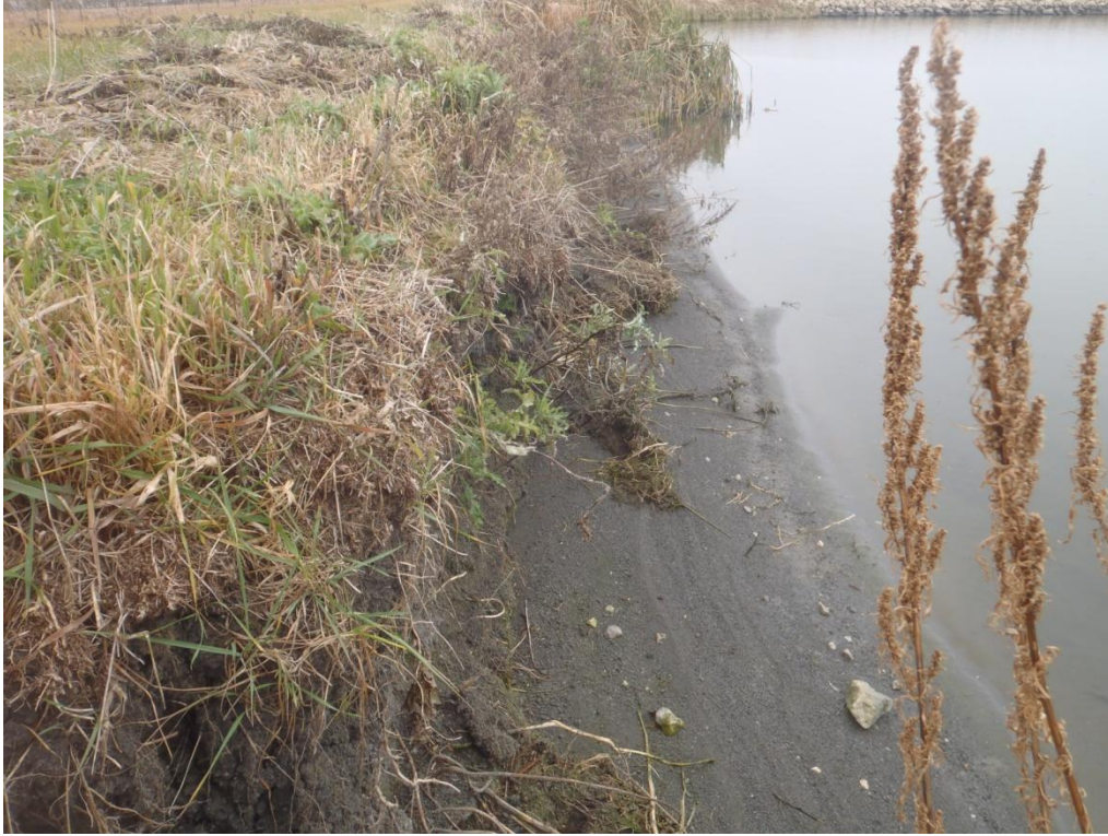
Photo 3: Erosion on north slope of primary cell
