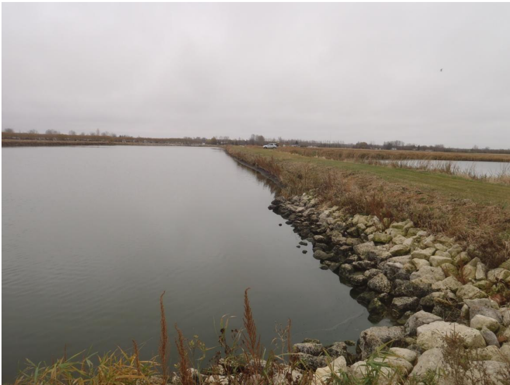
Photo 2: Erosion on south slope of primary cell
