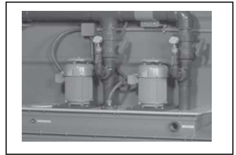
Dual Redundant Pumps
