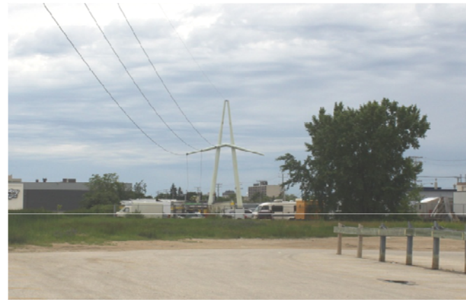
RS51 Transmission Line South of Station Site
