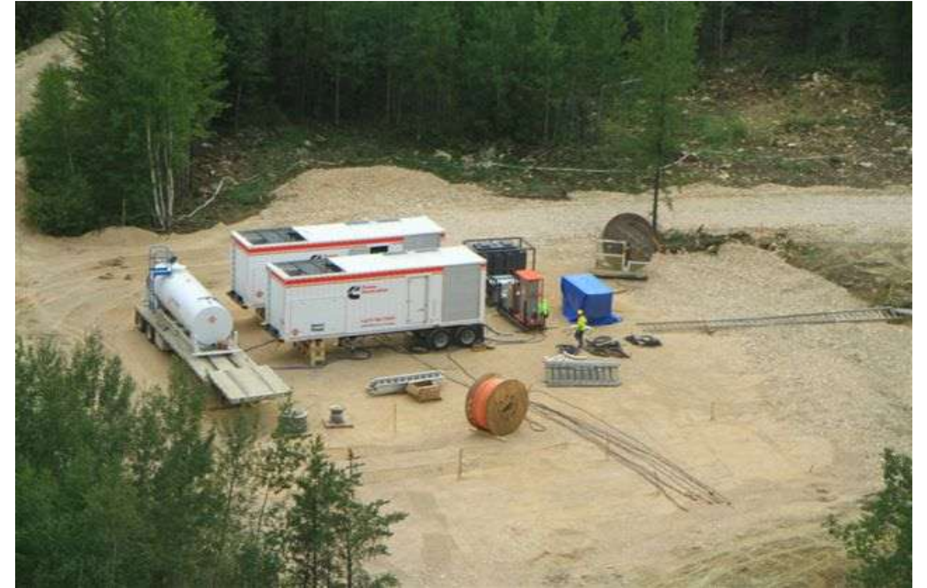
Generators and Power Lines
