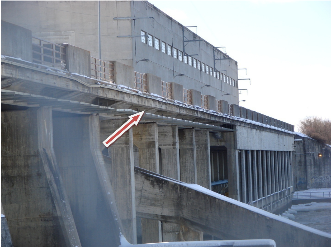
Figure 2-3: Cable Trays (indicated by arrow) on the Underside of PR #304 at the Pine Falls Generating Station
