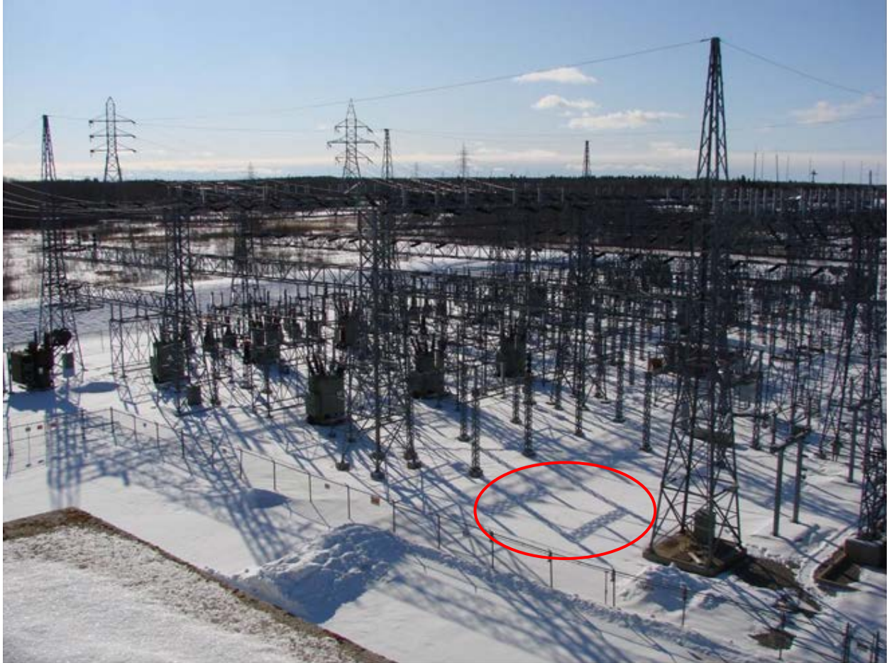
Figure 2-6: Pine Falls Generating Station Switchyard (Note underdeveloped area adjacent to the right hand foreground outlined in red)
