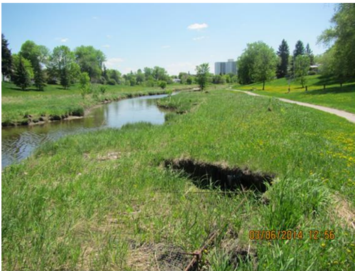
Figure 2.3 Bank failure and the remnants of the Aqua-Terra System on the west bank of Sturgeon Creek, downstream of the Ness Avenue crossing.
