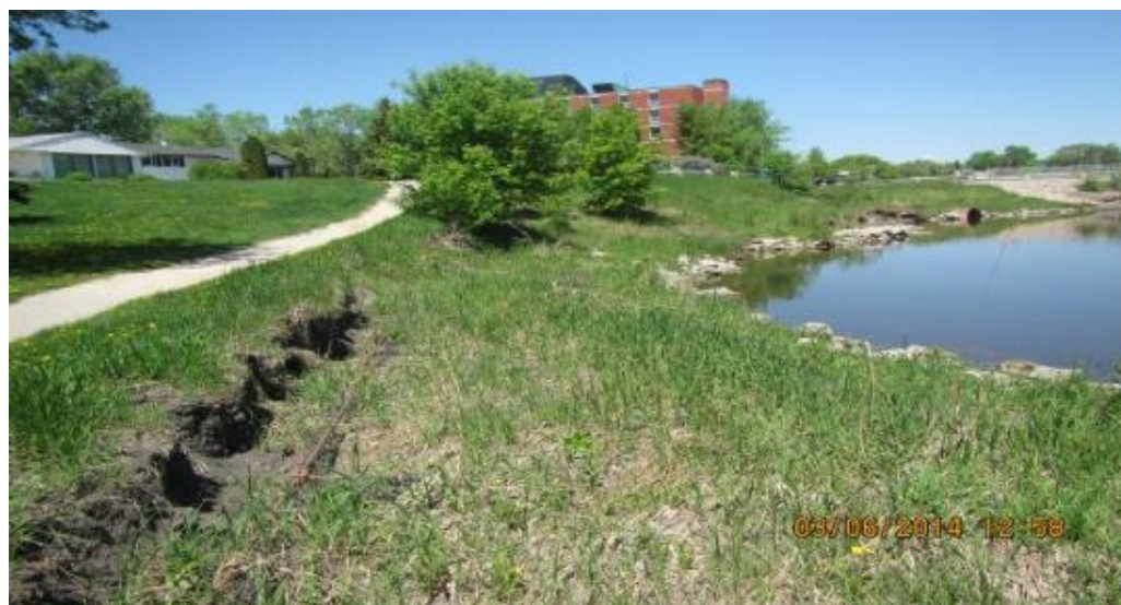
Figure 3.2 Slope instability on west bank, downstream of the Ness Avenue culvert.
