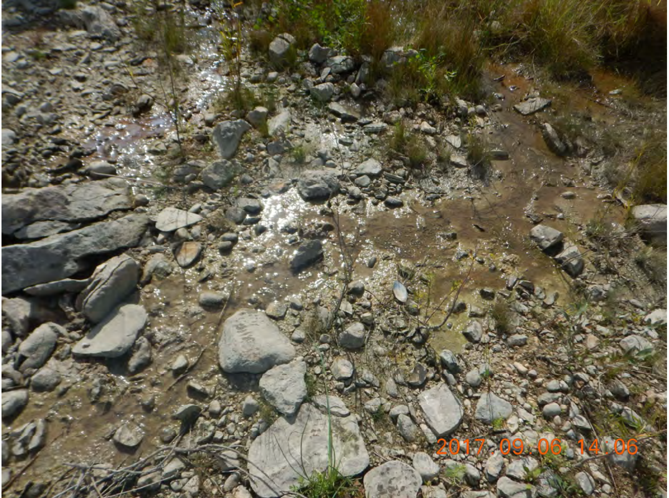
Photo 2: Slow seepage at additional discharge location.
