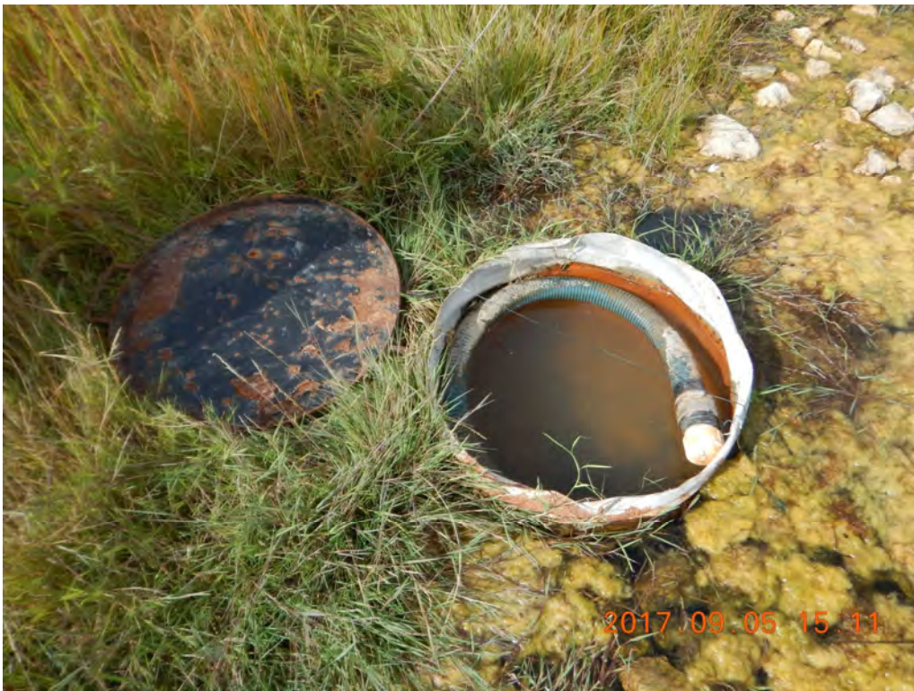
Photo 1: Low level sampling pipe and water within protective casing.
