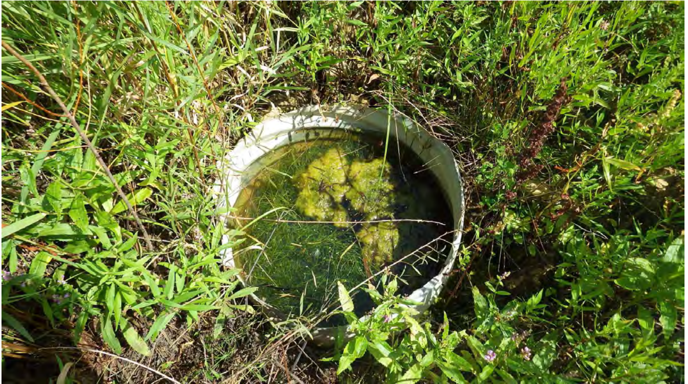
Photo 2: Low level sampling pipe and protective steel casing at 5A1. Cover is missing.
