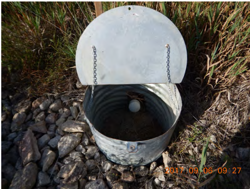
Photo 1: High level sampling pipe and protective CMP casing.
