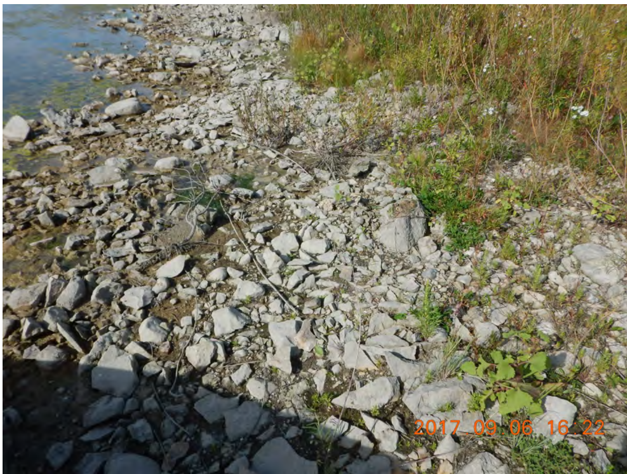
Photo 2: Low flow seepage into channel.
