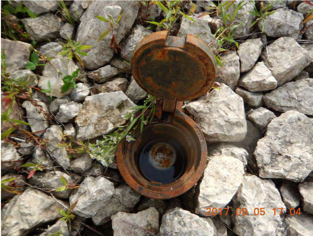
Photo 2: Low level sampling pipe and protective steel casing at 8C1.
