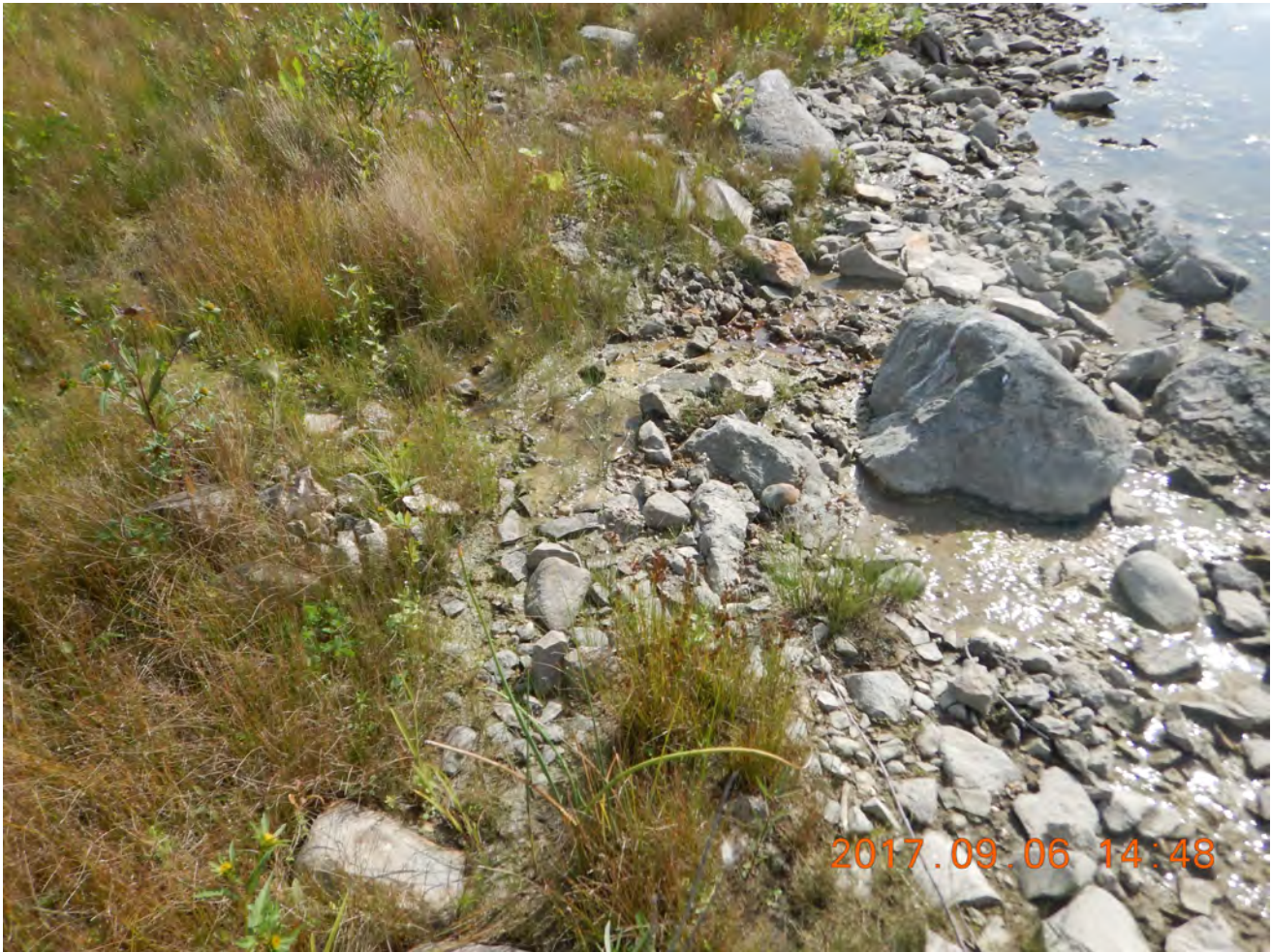
Photo 2: Low flow seepage into channel.
