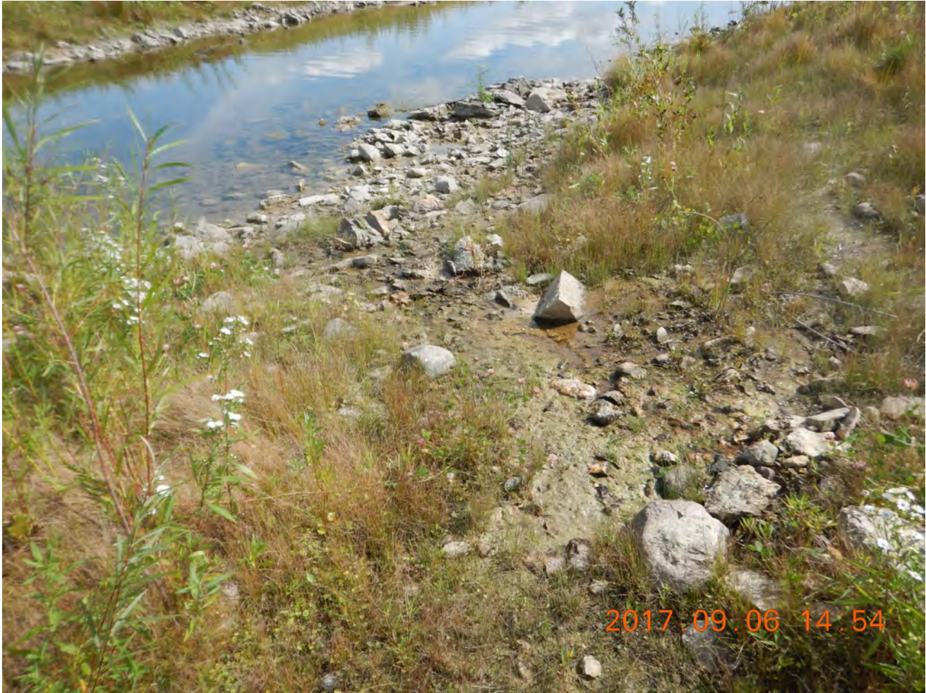
Photo 2: Low flow seepage into channel.
