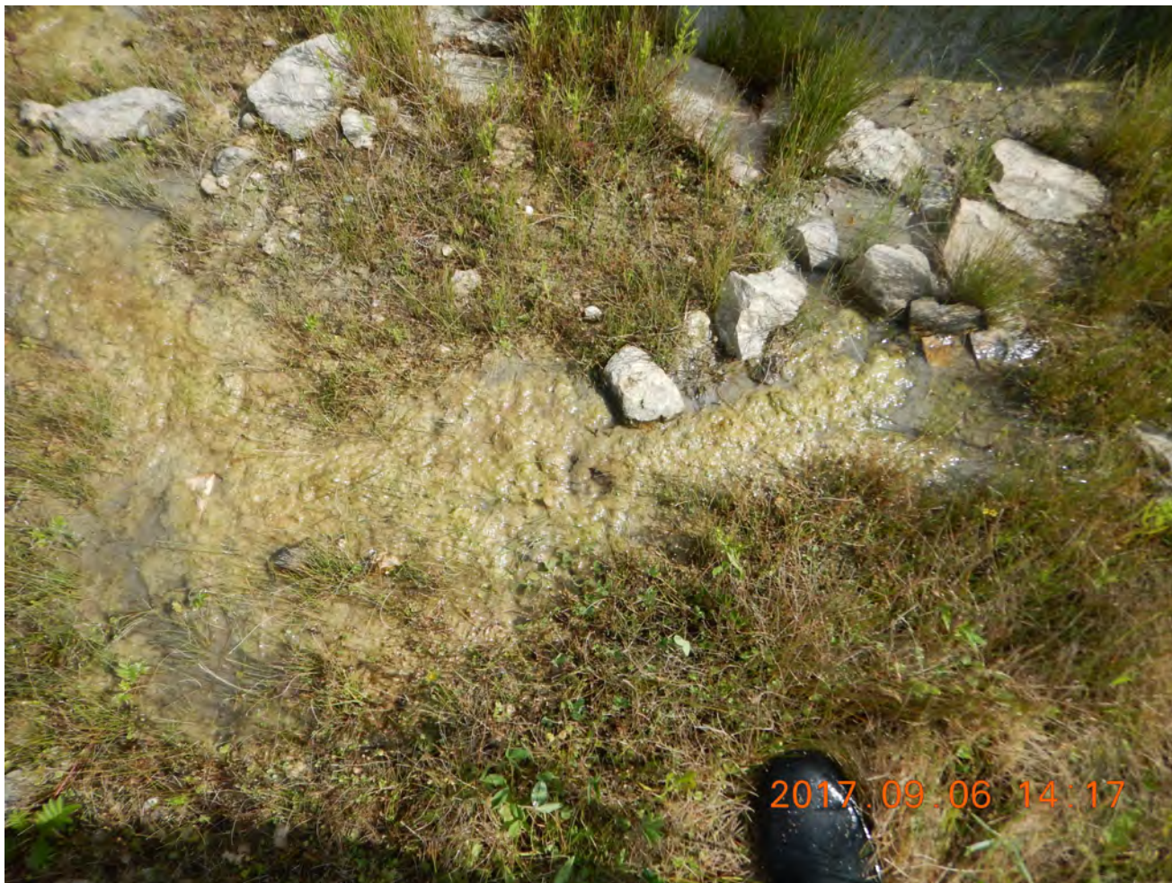
Photo 2: Slow seepage at additional discharge location.
