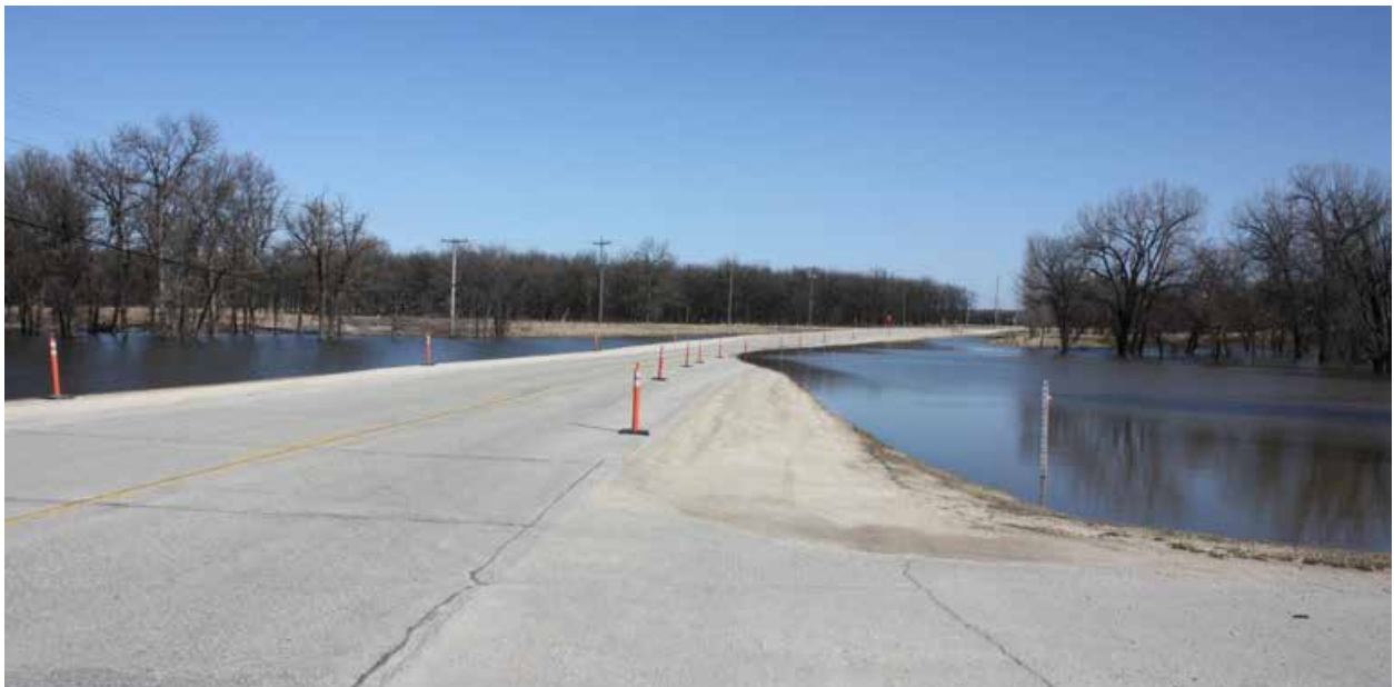
St. Mary's Road North of Richardson Road, Flooding April 13, 2011
