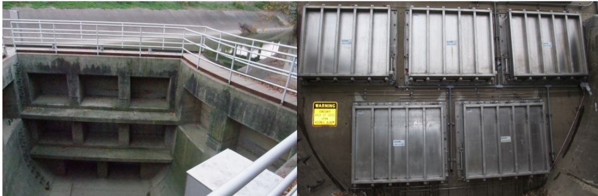
Figure 3-2. Example ACU-GATE Installation (Picture credit: courtesy of Grande, priv comm 9/11/2018)
