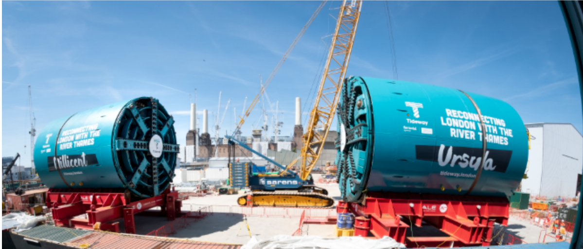
Figure 7-2. Two TBMs Currently Being Used in the Thames Tideway Project in London, UK (Picture credit: https://www.tideway.london/the-tunnel/the-engineering/ )
