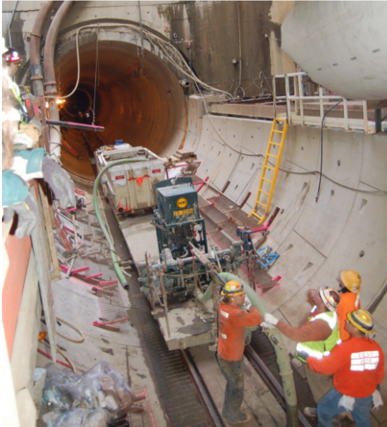
Figure 7-4. West Side CSO Tunnel Under Construction in Portland, Oregon (Picture credit: https://en.wikipedia.org/wiki/West_Side_CSO_Tunnel )
