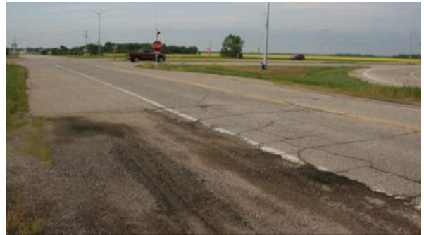
Gravel shoulder deterioration on the north leg
