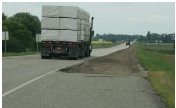
Gravel shoulder deterioration on the south leg
