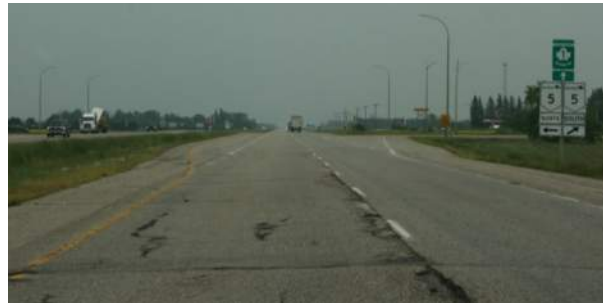
Pavement cracking on the eastbound approach
