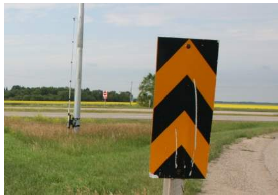
Example of Sign Deterioration
