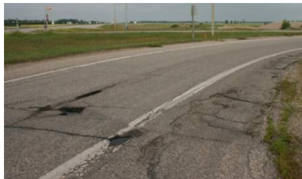
Pavement cracking at the right-turn channel at the northeast corner
