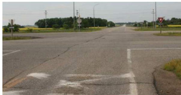
Pavement cracking at intersection (facing south)
