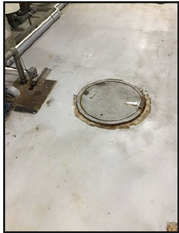
Figure 11. Chill Water Room Pit
