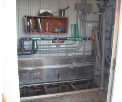
1.2 Interior of SBR building with sewage influent transfer piping
