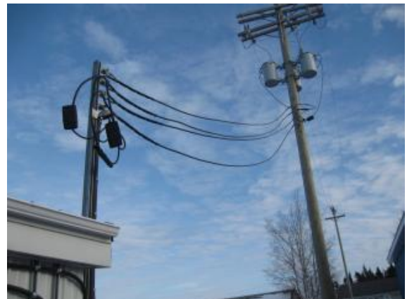
1.6 Electrical service to UV building
