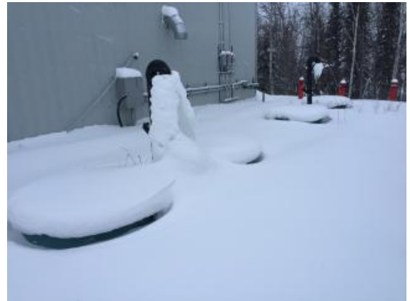
1.10 Sludge digestion underground tanks
