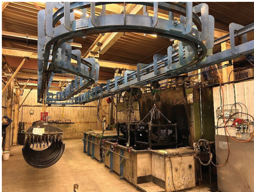
Figure 2-1 Parts Conveyor and Paint Tank in West Shop Paint Room
